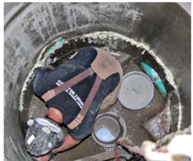
Studies show that 40 percent of groundwater infiltration in sewer systems enters through manholes.
