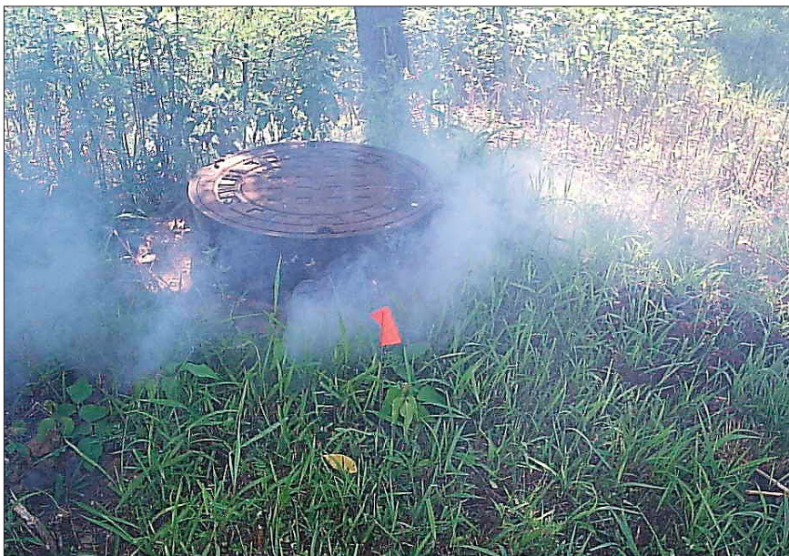
Smoke testing reveals a manhole defect in need of attention.
